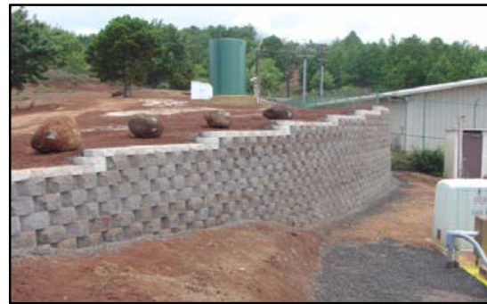
Erosion Control at Mākaha Ridge Tracking Station
